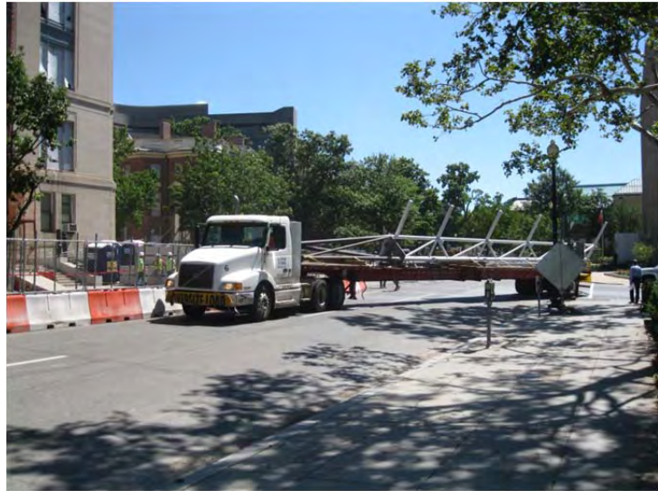
Figure 17: Atrium Built-Up Truss Column Delivery on the intersection of 18 th Street NW and E Street NW – Courtesy of the Whiting-Turner/Walsh Joint Venture
