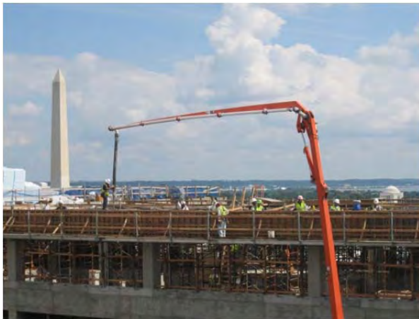
Figure 2: Pouring of the roof slab of the New Addition – Photo Taken by Ramuel Holgado
